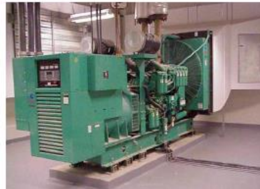
Generator or the other machines
