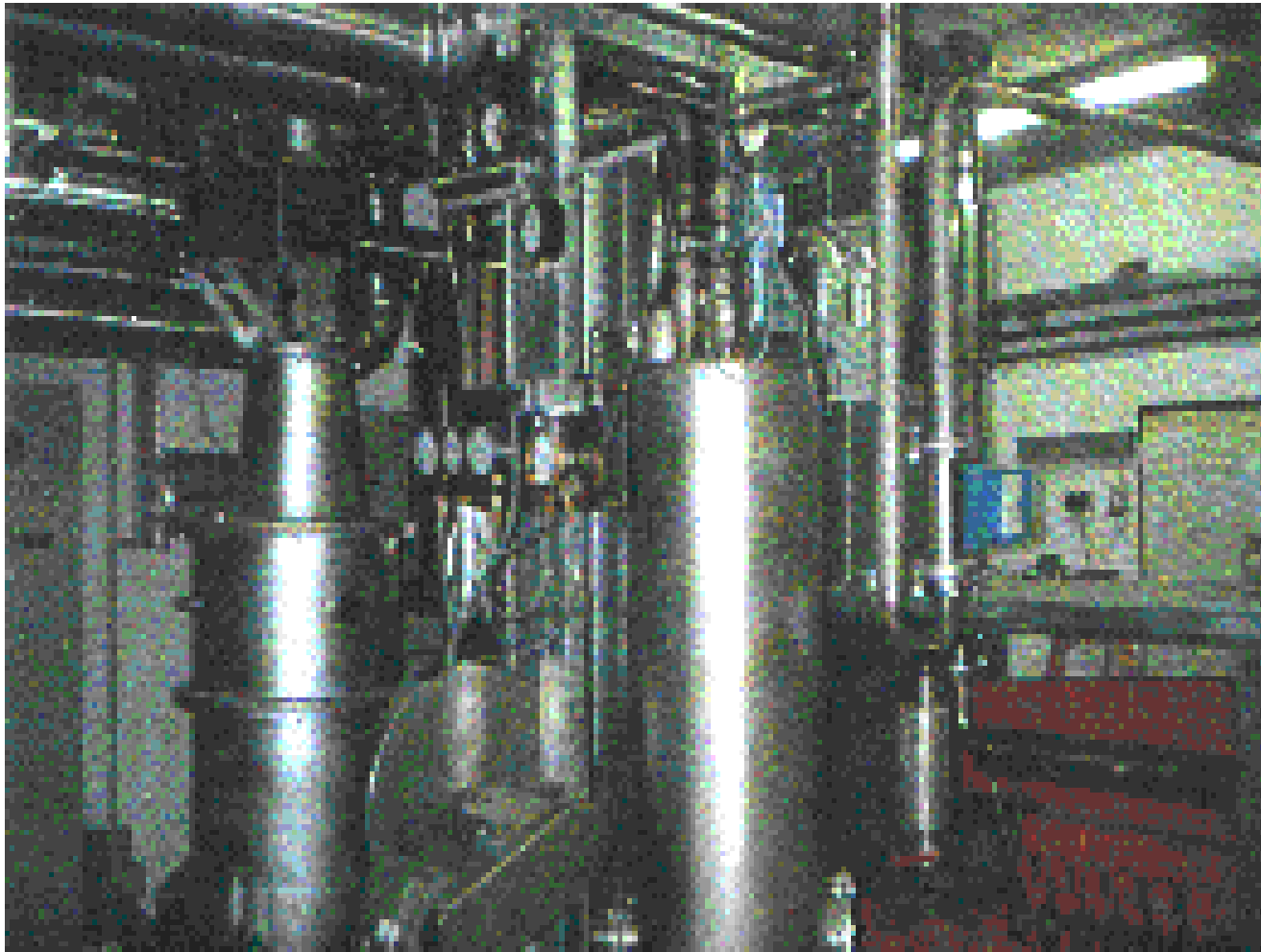
Wood gasifier for co-gen set
