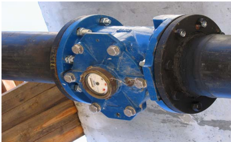
Figure 6.4 Measuring pumping rate by flow meter
