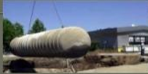
Leaking Fuel and Chemical Tanks
