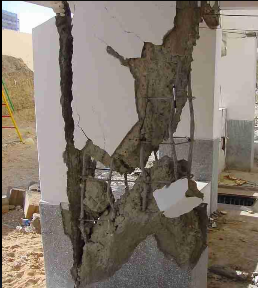
Diagonal cracks in columns
